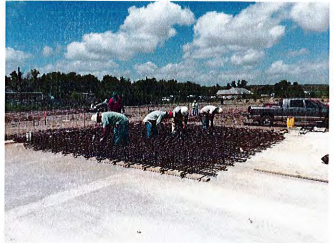
Workers are tying rebar for the paving on the western edge of the site.
