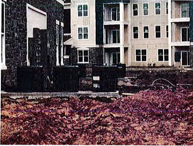
Condensing units had been installed around the buildings.
