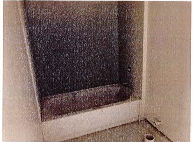
Bathrooms had tubs installed and drywall was substantially complete with painting substantially complete.
