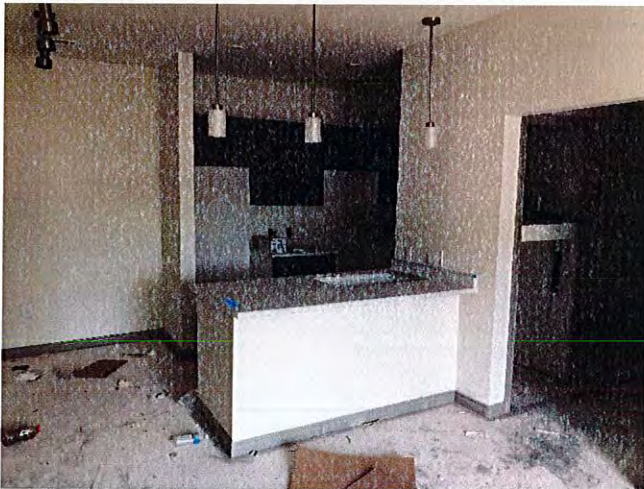
View of the interior at building 1 with countertops and cabinets in place.
