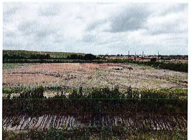
Overall view of the cricket field which had excavation operations substantially complete.
