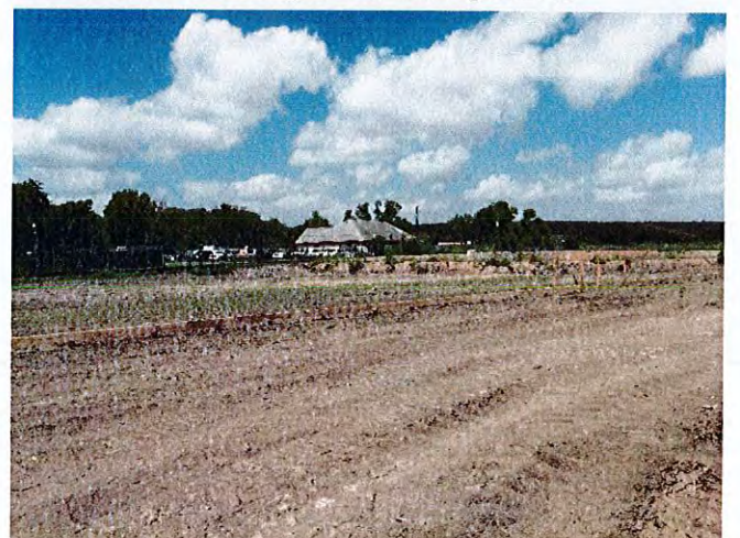
Grading and formwork for the paving is underway at the west side of the site.
