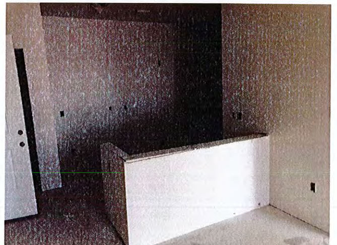
View of the kitchen of a unit in building 5 with drywall in place.
