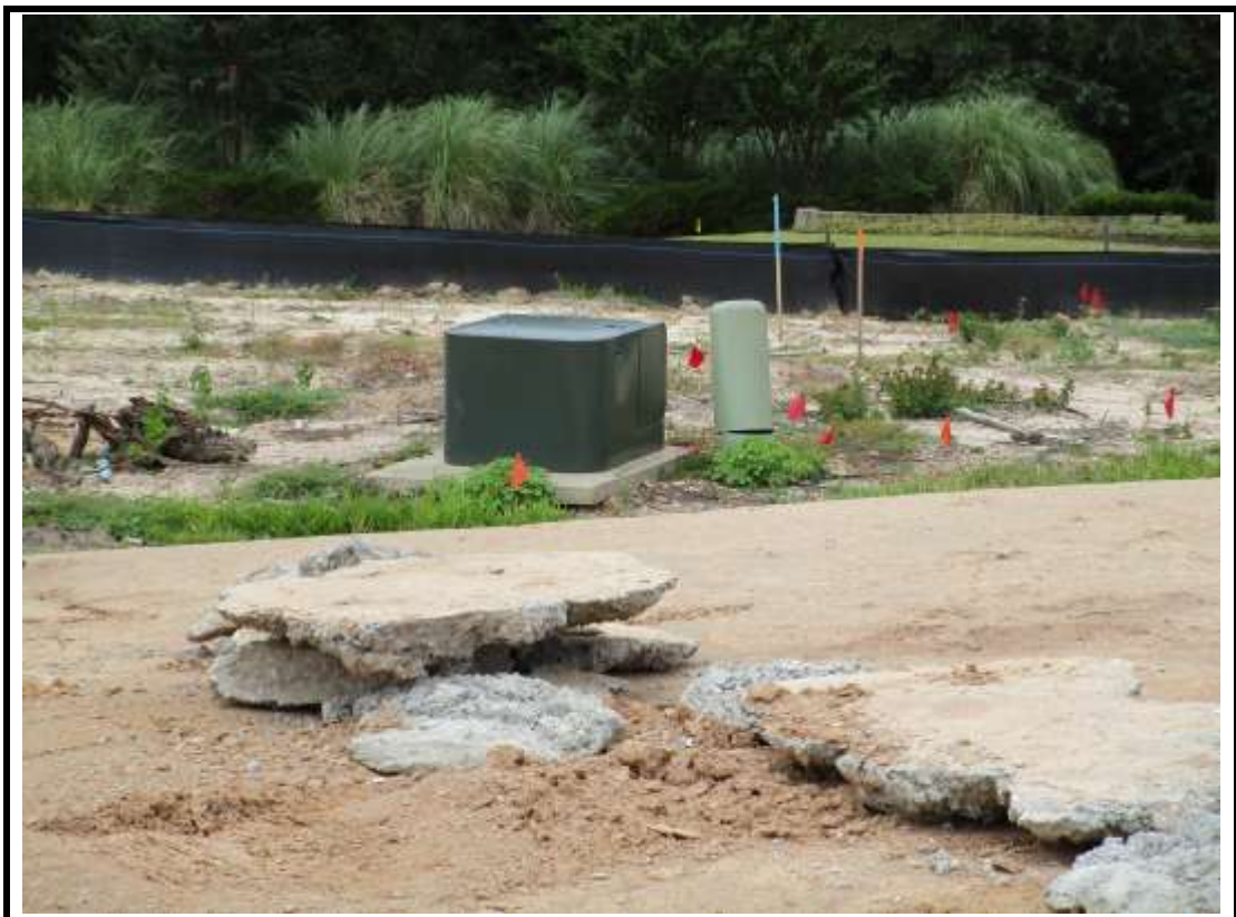
Photograph 12: Transformer to neighbor's house to be relocated this week.
