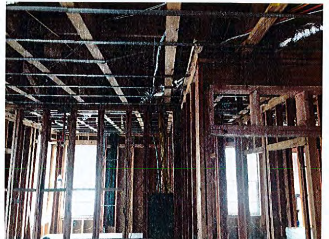
The installation of the electrical wiring and HVAC was nearing completion at Building #2.
