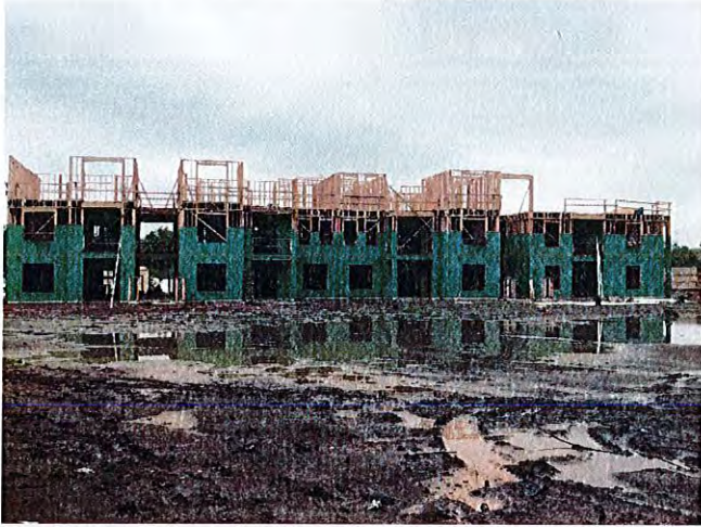
Rough framing operations were in progress on the third floor on building 3.
