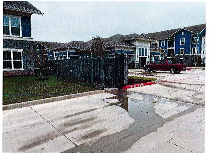
View of the gates which had been installed at the north end of the job site.
