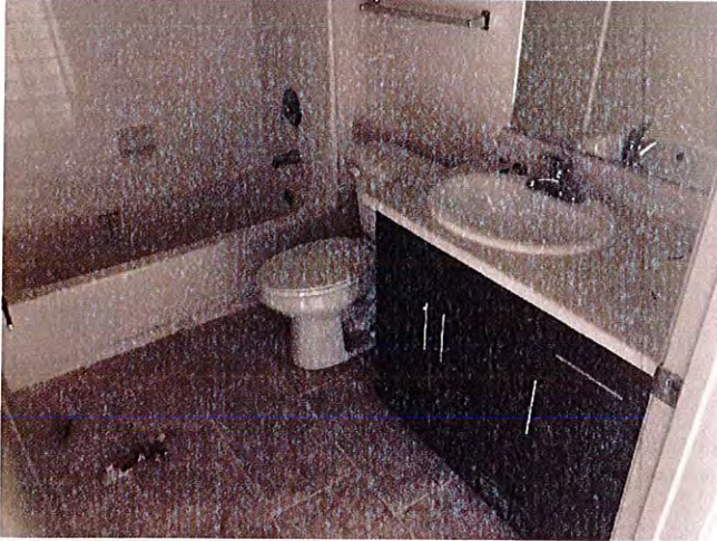
Sinks, toilets, tubs and floors had been installed at the bathrooms at building 1.
