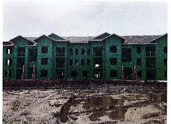
The installation of the roof was substantially complete on all the Buildings.
