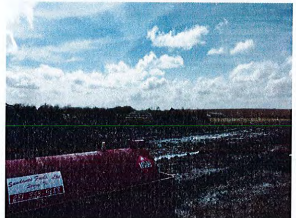
4. The site will be cleared of the trees, shrubs and stumps next week.
