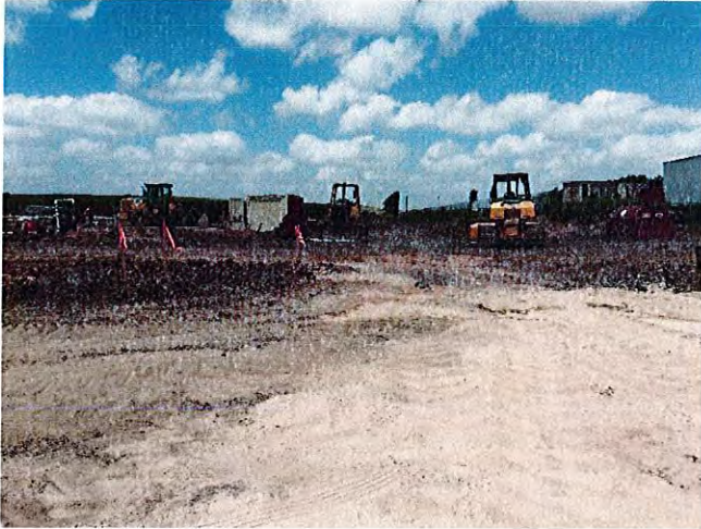
Grading at the southeastern edge of the property for the paving was underway.
