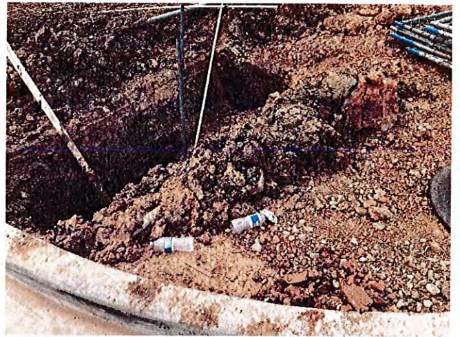
View of the concrete curbs in place and the clean up process that was substantially complete.
