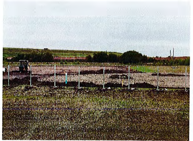
View of the cricket field with the fence around the perimeter being installed.
