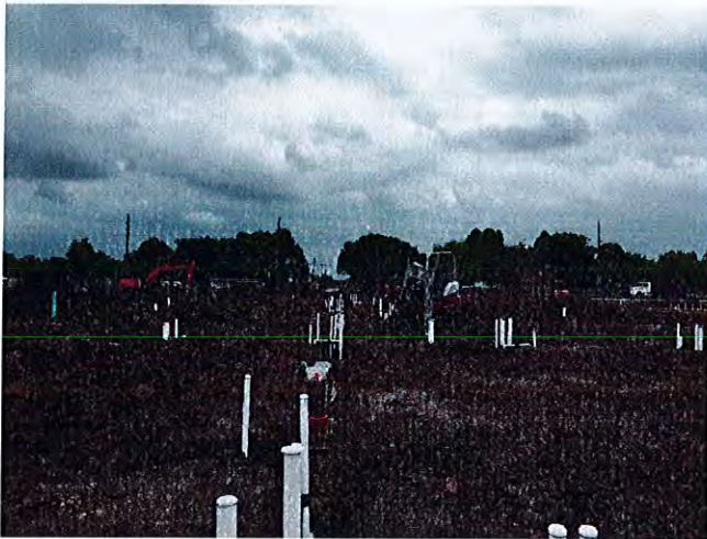
Excavation for the underground utilities is underway at building 1 and the clubhouse.
