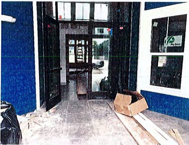
View of the storefront entrance to the clubhouse with doors and windows in place.
