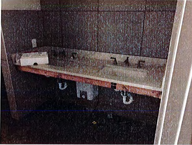
View of the sinks which had been installed at the clubhouse.
