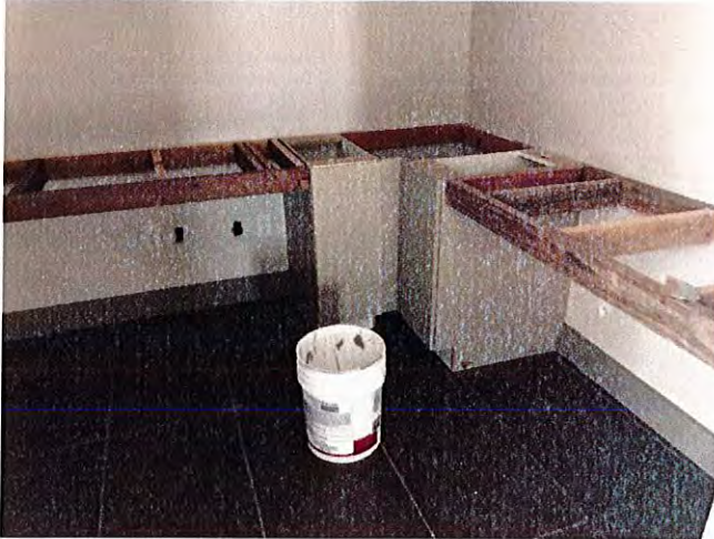
Cabinets were awaiting installation at the clubhouse.
