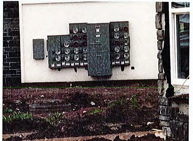
New electrical meter bank had been installed at building 5.
