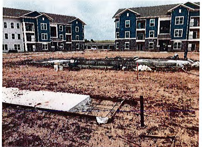
Overall view of two buildings and the concrete pool which was being installed in the courtyard.
