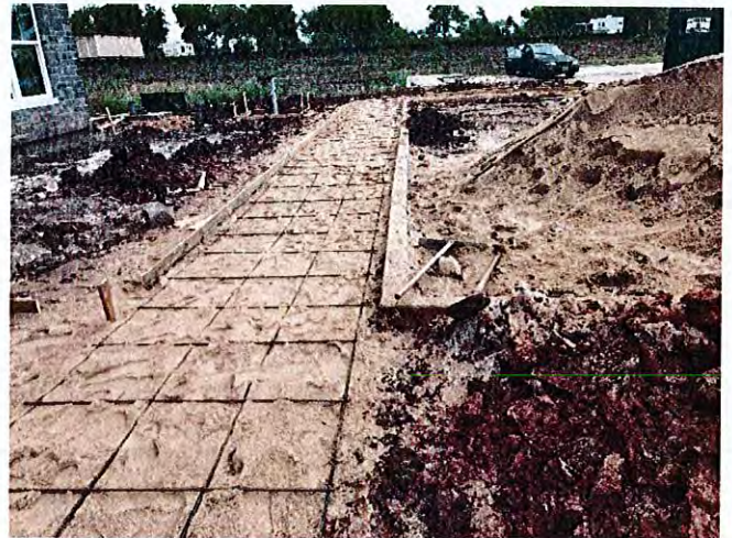
Overall view of reinforcement in place for the sidewalks to be installed.
