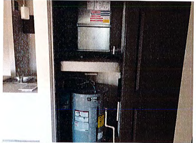
HVAC and hot water heater units were in place at building 1.
