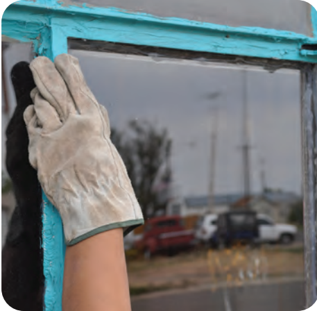
5. Install new glass, using tempered where code requires, that meets or exceeds previous glazing
