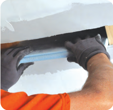
5. Blocking still needs to be put into place
