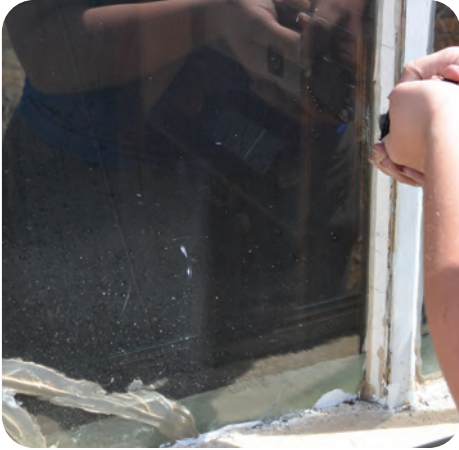
1. Remove all broken glass
